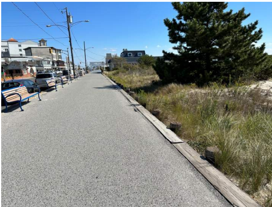
Photo #18 - Settlement behind failing timber bulkhead.
