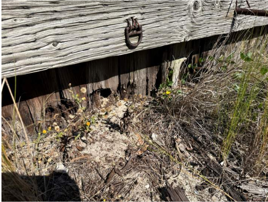
Photo #17 - Failing timber bulkhead on south side of the promenade on the West End.
