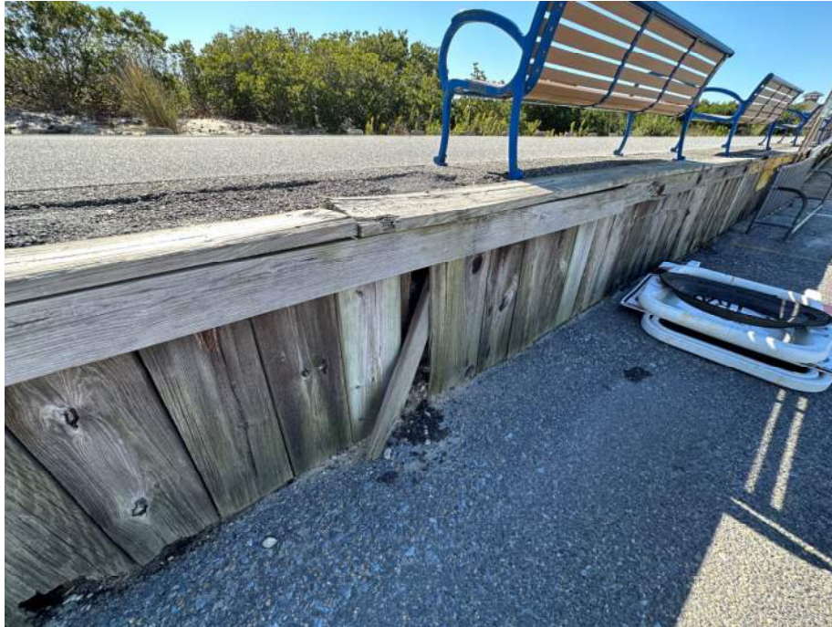
Photo #21 – Failing timber bulkhead on along Beach Avenue.
