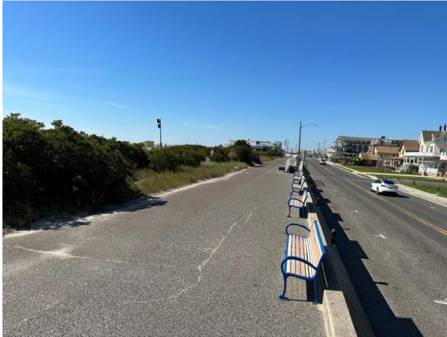
Photo #11 – Asphalt walking surface. Fair conditon.
