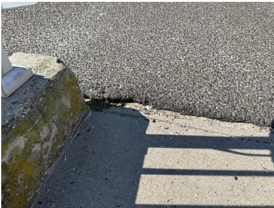
Photo #6 – Tripping hazard at top of ramp.
