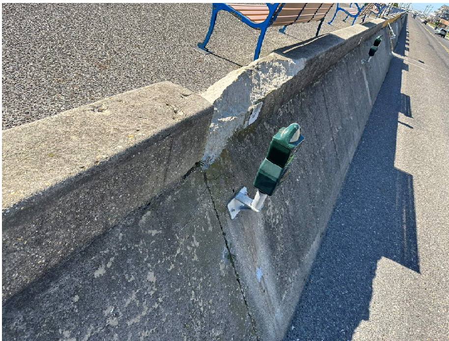
Photo #8 - Large concrete spall.
