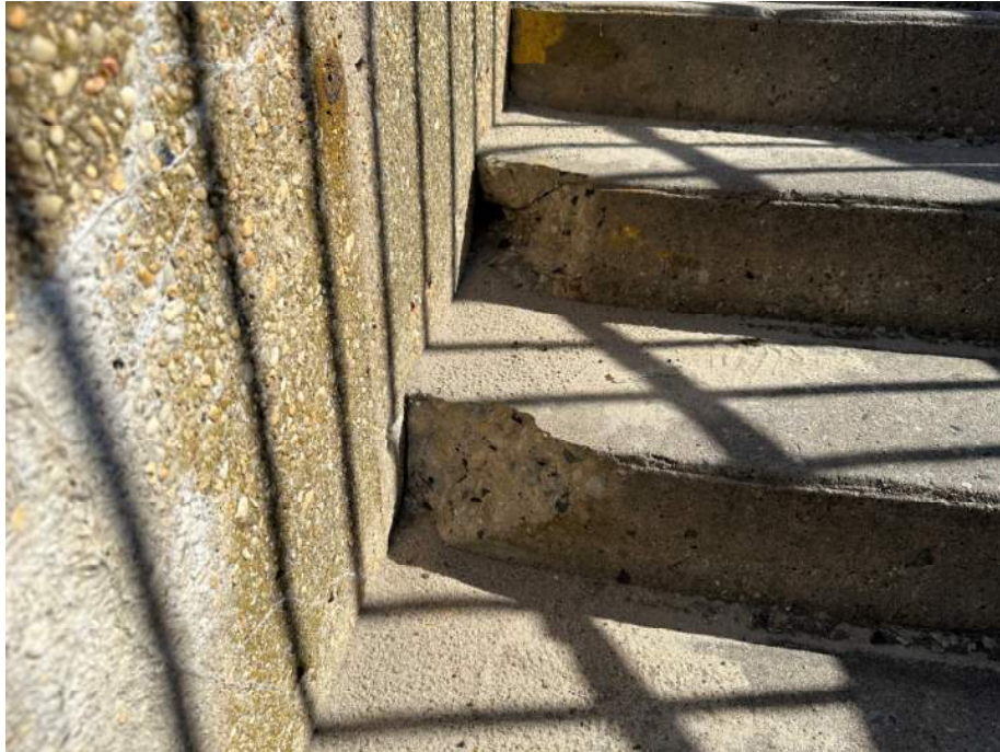
Photo #3 - Deteriorated concrete steps.
