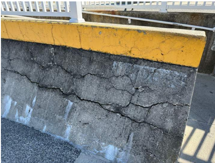
Photo #14 – Concrete cracking and delamination.
