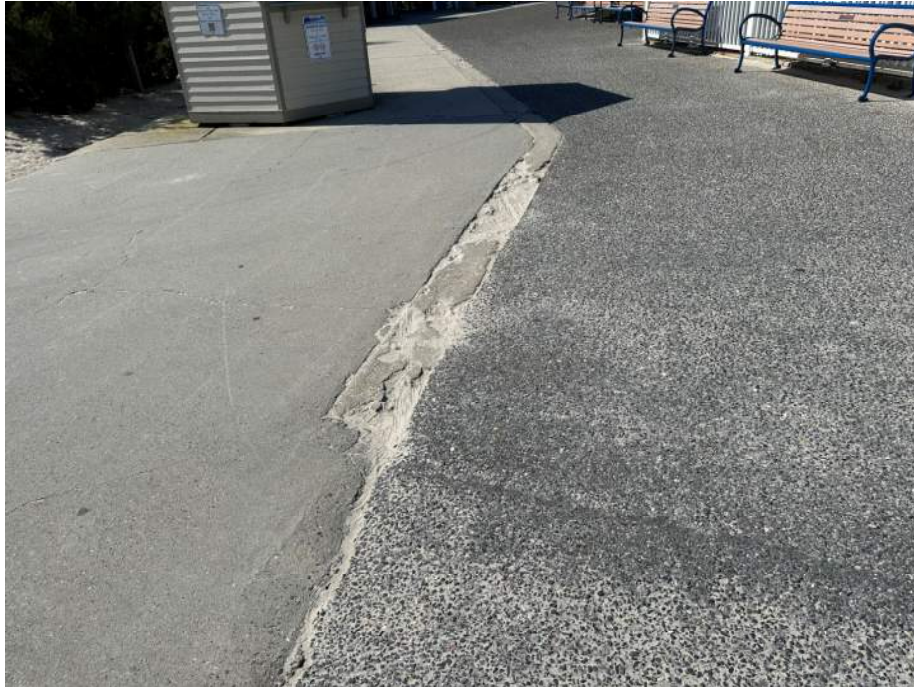
Photo #13 – Tripping hazards on promenade.
