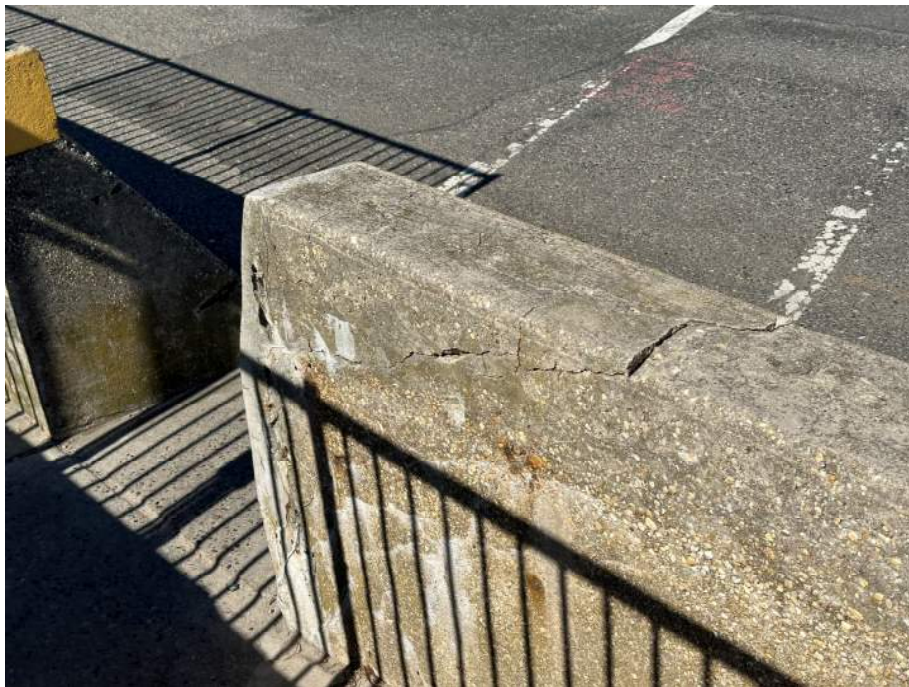
Photo #2 – Concrete deterioration on Madison Ave.
