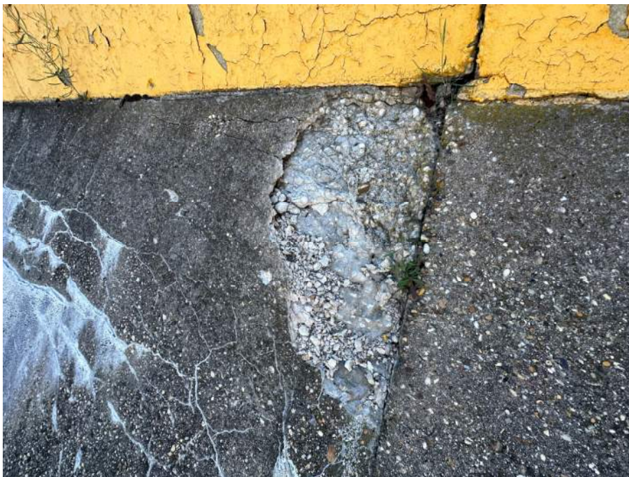
Photo #10 – Concrete cracking and delamination.
