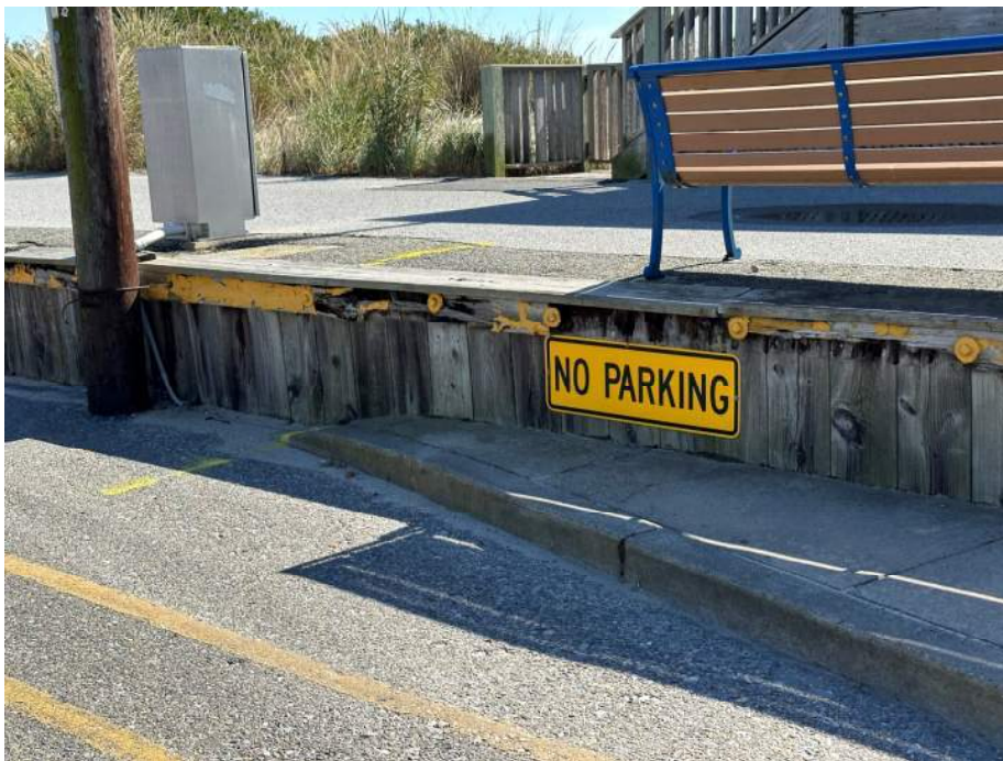
Photo #22 – Failing timber bulkhead along Beach Avenue.
