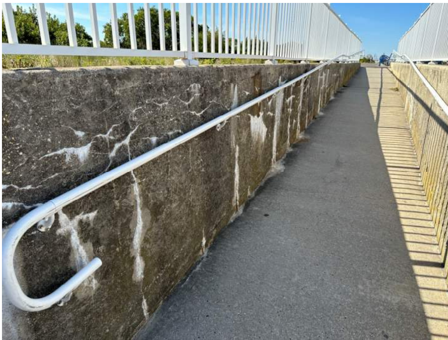
Photo #4 - Efflorescence on ramp walls.
