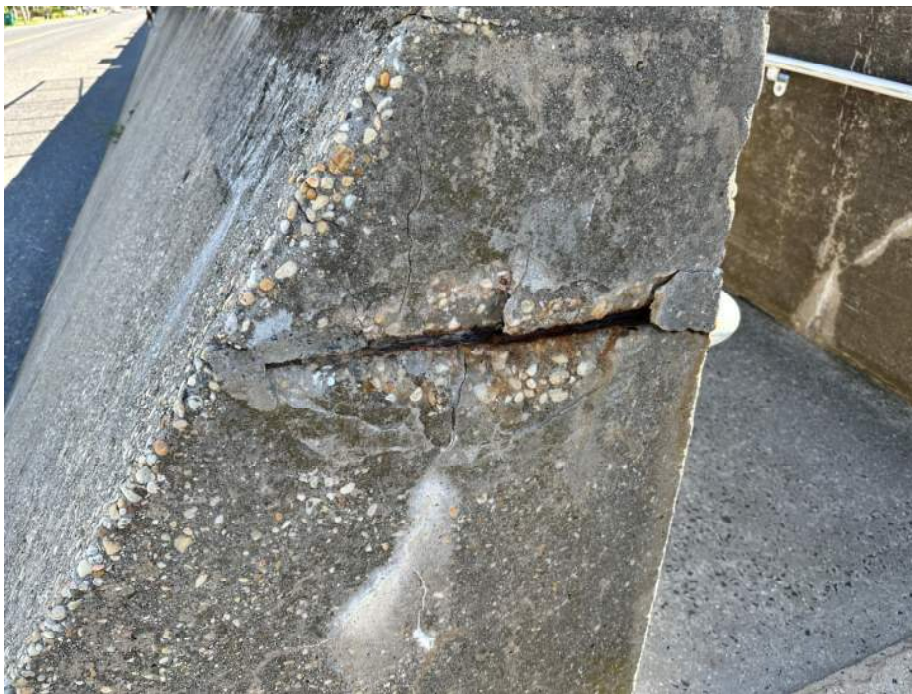
Photo #12 – Concrete spalling and exposed rebar.
