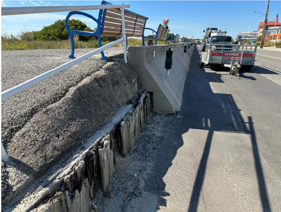
Photo #1 – Deteriorated timber bulkhead at Promenade East End.
