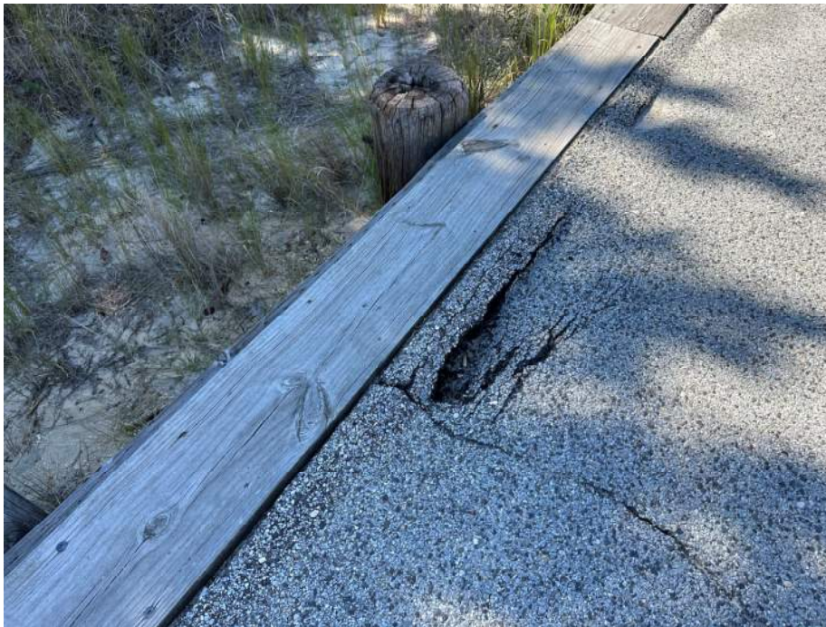
Photo #16 - Sinkhole formation behind failing timber bulkhead.
