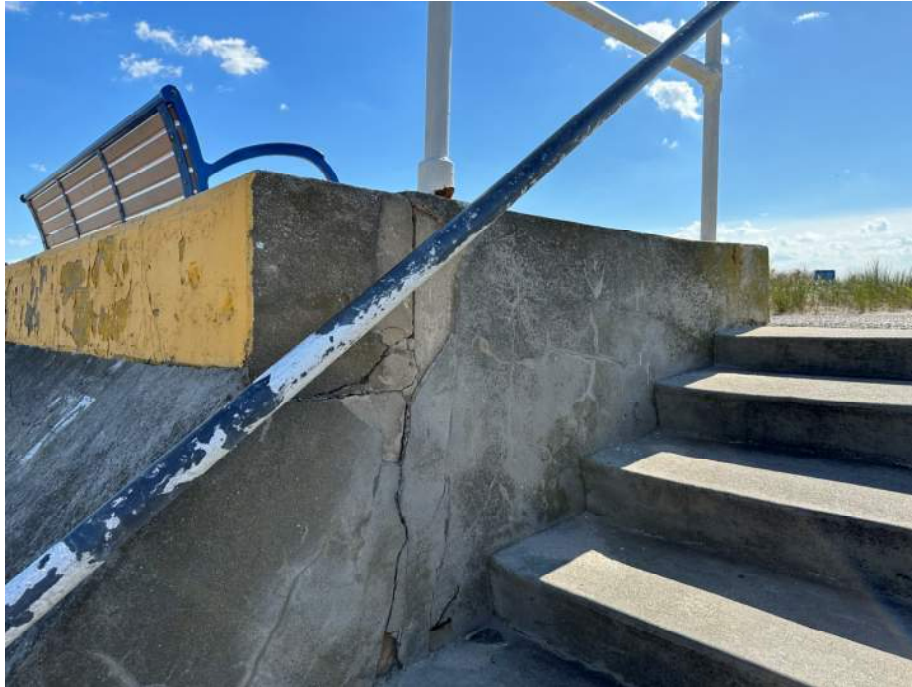
Photo #9 – Concrete cracking and delamination.
