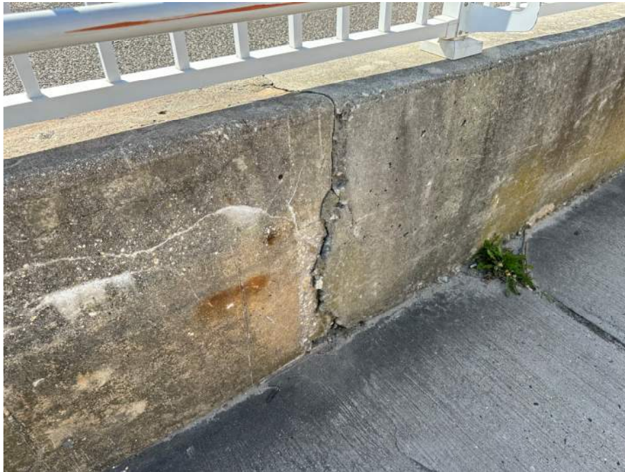
Photo #5 – Deteriorated concrete.
